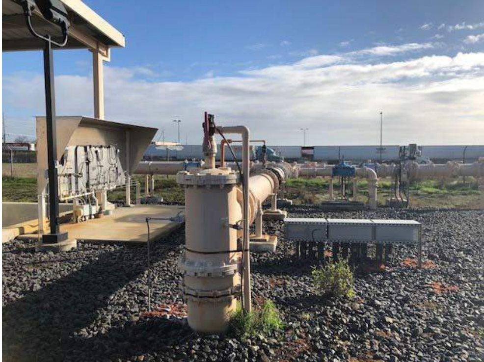
PHOTOGRAPH 3.1-4: LOUISE AVENUE WATER TREATMENT FACILITY BLENDING INFRASTRUCTURE
